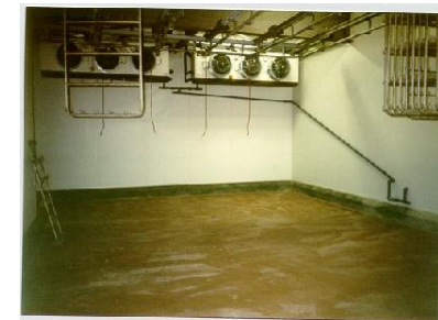
Carcass Chiller with rails
