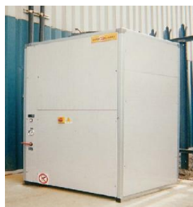
Process water chiller
