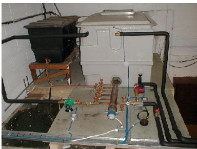
Heat Recovery System
