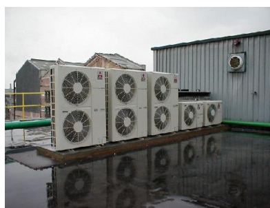
External condensing units
