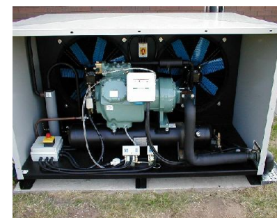
Condensing unit in housing
